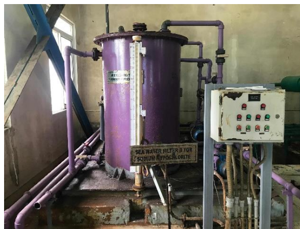
Gambar 3. Sea Water Tank Sodium Hypochlorite
