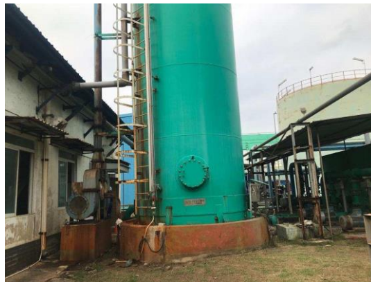
Gambar 6. Tank Sodium Hypochlorite
